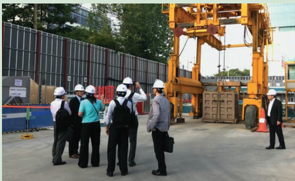
[CEO of WHC and 20 officials from the MOH visiting the site (June 8, 2017)]
